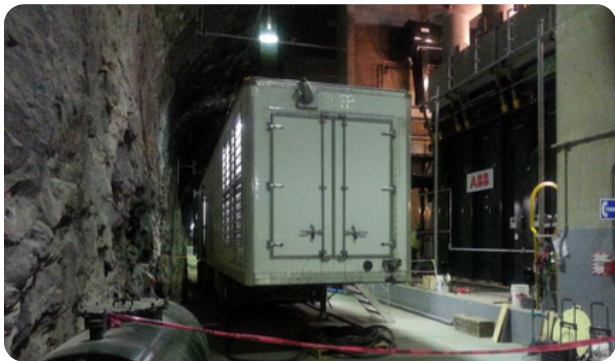
Above: TORS-6000, at underground generating station
